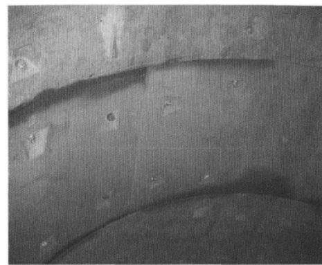
Segment cracking and water seepage of Chengdu Metro Line 1 caused by Wenchuan Earthquake
