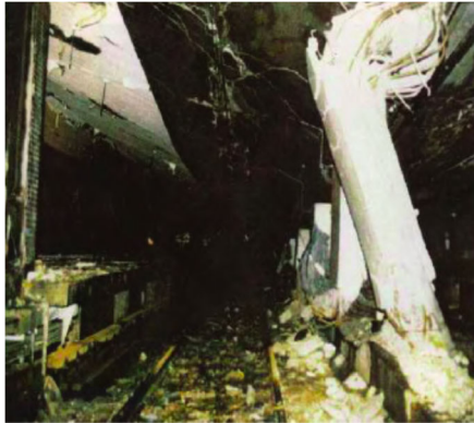
The central column collapse of Daikai Station after the Hanshin Earthquake in Japan
